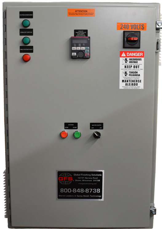
Figure 2. BNP control panel on a booth with manual balance
