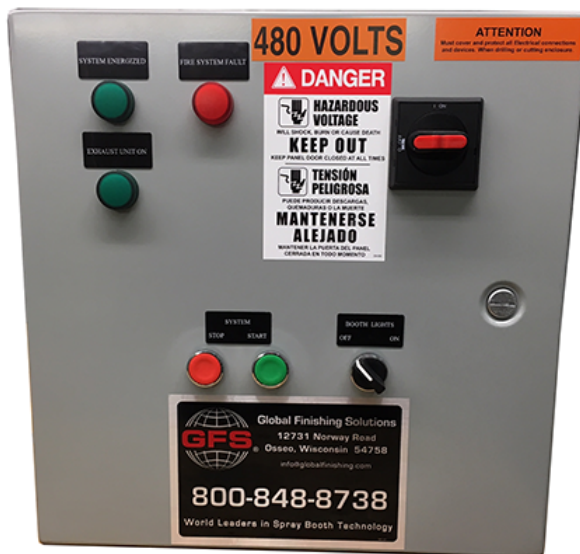
Figure 1. BNP control panel
